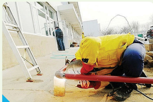
A Langfang Gas employee changes the gas pipeline at the designated hospital
