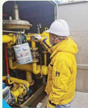
Leakage detection of the Roots flowmeter at the Central Hospital of Qingdao West Coast New District
